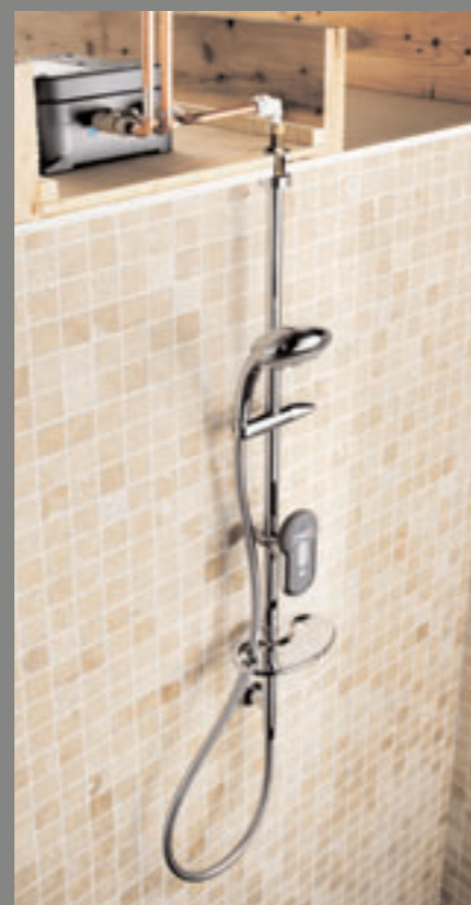
▲ Loft installation – convenient for water inputs and ceiling connection to shower
